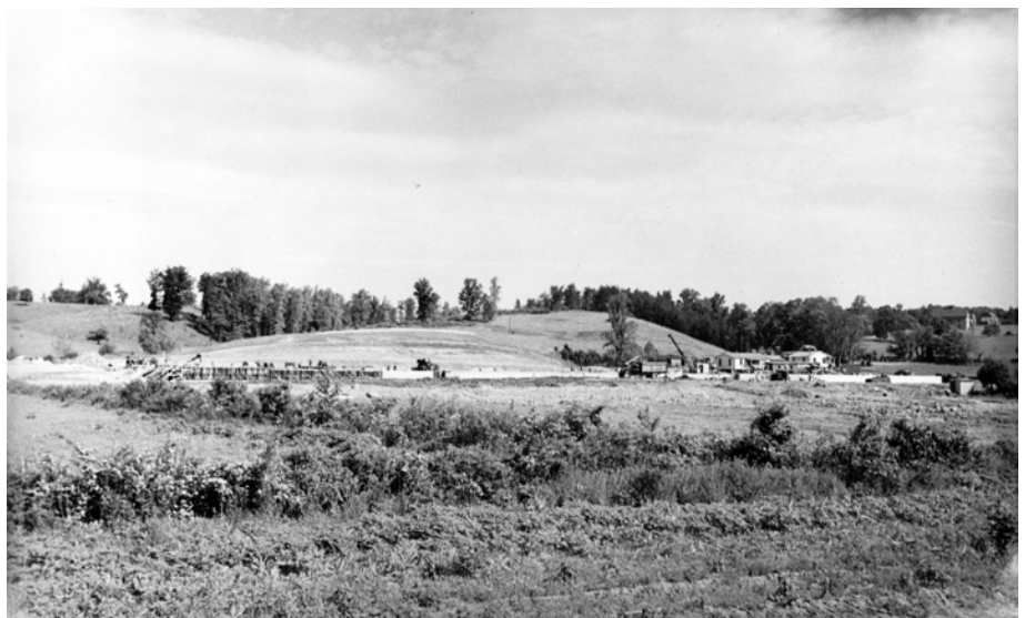
This photo was taken on May 18, 1944, looking north at the plant construction in process from the C&O Railroad track.
