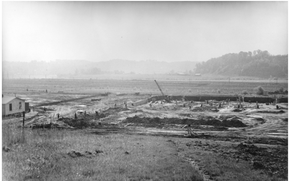
Excavation at the U.S. Rubber Plant site began in early 1944 at a site just west of Scottsville. This photo was taken circa April 1944, looking south at the plant site with the James River in the background.
